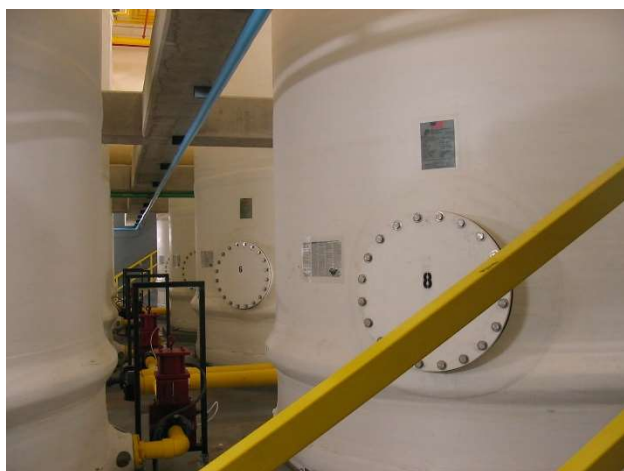
Figure 5 – Large Disinfection facility (USA)
