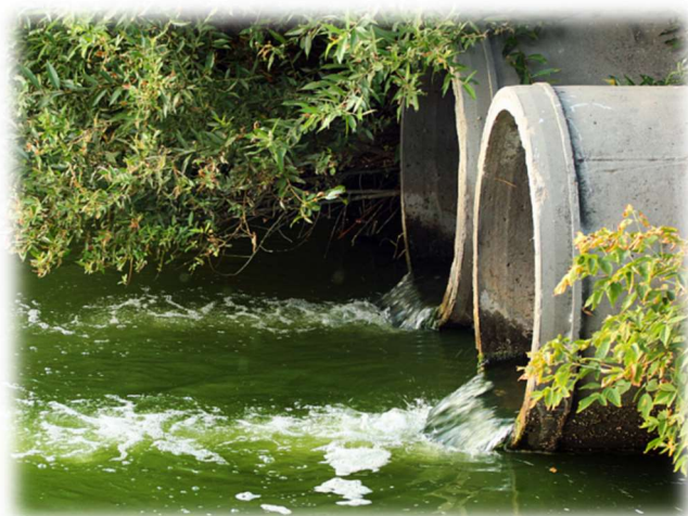
Figure 1- Overflow discharging into watercourse.
