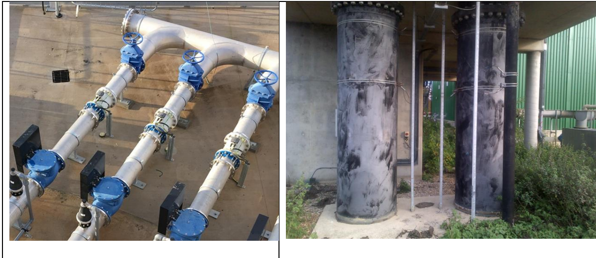
Figure 4. Pass forward flow meters at sewage pumping stations.
